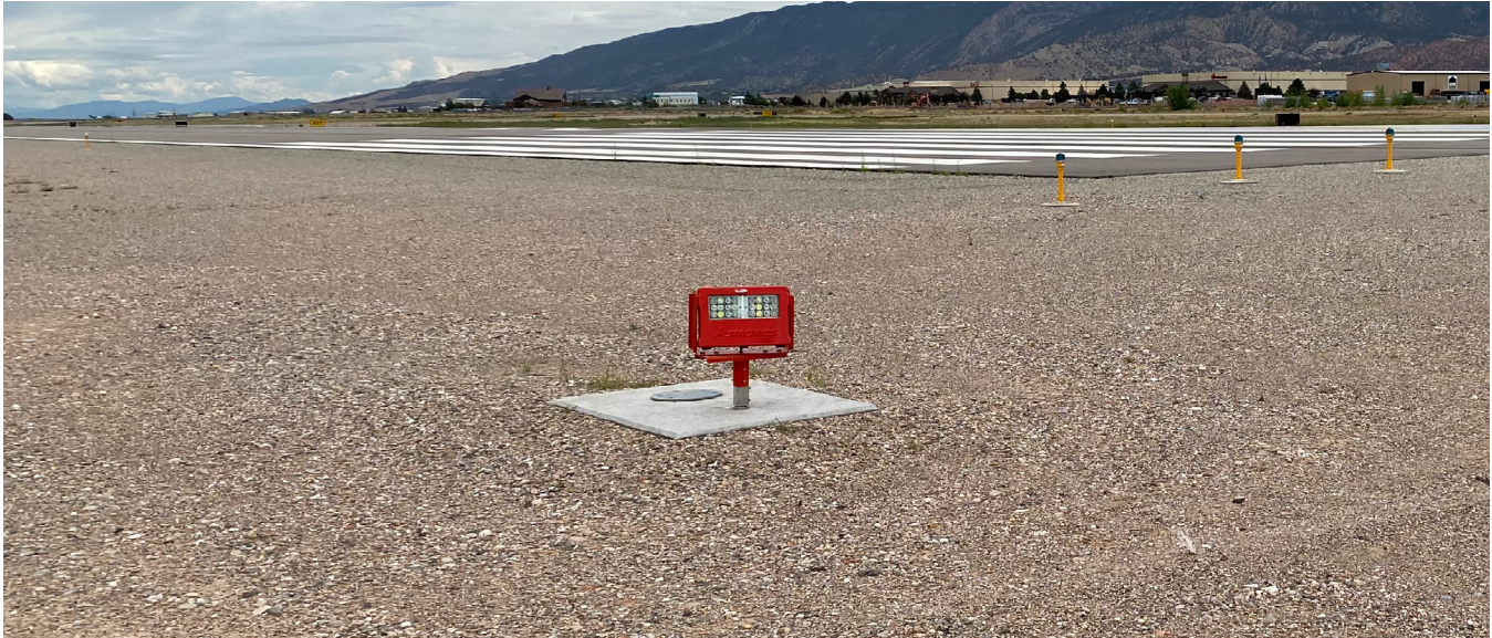
Figure 4.12: Runway End Identifier Lights
